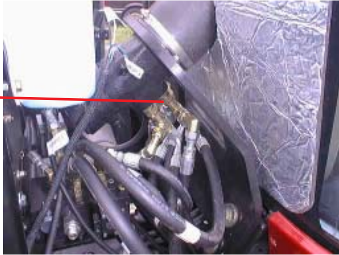
Tank hose connection to orbital tee fitting
